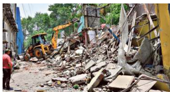
Illegal constructions being demolished during the anti-encroachment drive on Wednesday. • R.V. MOORTHY
