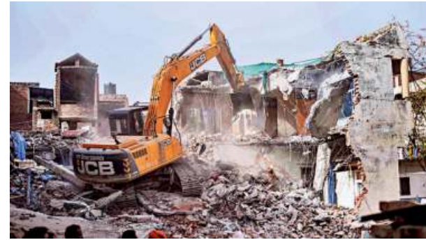
Brought down: A bulldozer being used to demolish the bungalow of an activist in Prayagraj on Sunday. ■ PTI
