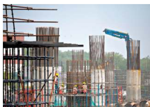
Stable growth: Workers assemble metal rods to make a concrete pillar at a flyover construction site in New Delhi. ■ AFP
