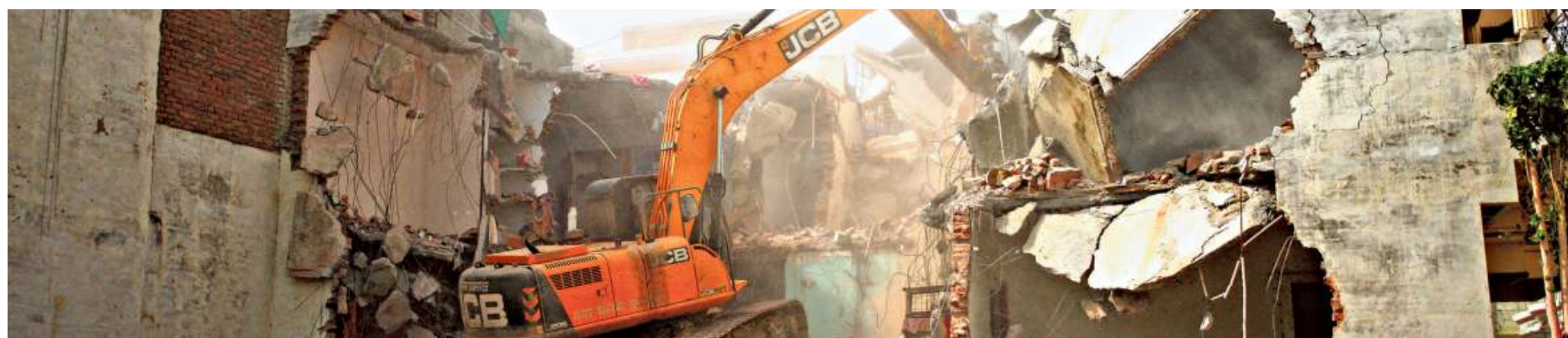
In ruins: A bulldozer demolishes the house of a Muslim man, who Uttar Pradesh State authorities accuse of being involved in riots, in Prayagraj on June 12. • REUTERS
