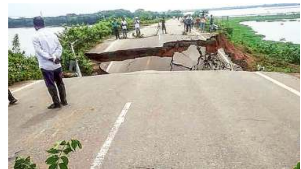
Lifelines snapped: A road damaged in floods in Karimganj district on Friday. •PTI
