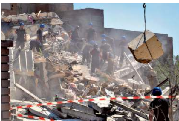
Sifting through rubble: Ukrainian rescue officials clearing debris at a damaged building in Serhiivka on Saturday. • AP
