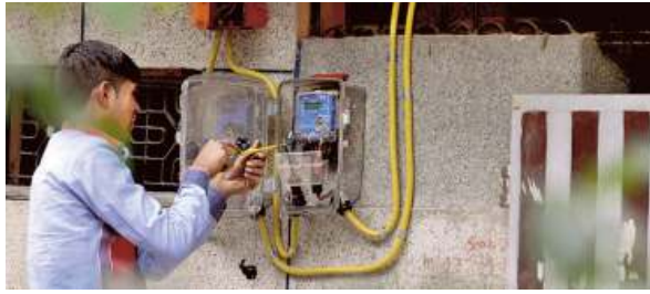
The smart meters will allow consumers to monitor and analyse their power consumption. • FILE PHOTO
