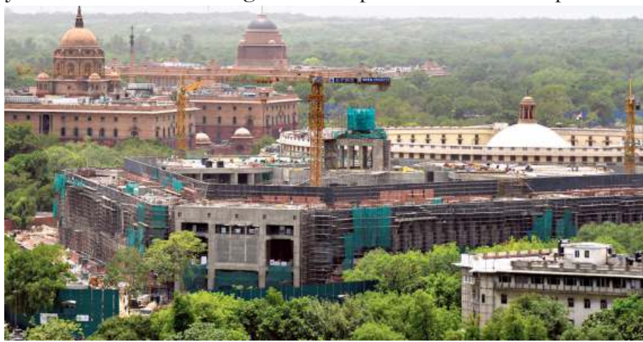
Changing face: Work in full swing on the new Parliament building complex under the Central Vista redevelopment project in New Delhi on June 9. •R.V. MOORTHY
