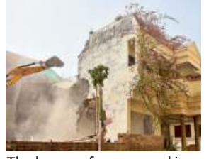
The house of an accused in the Prayagraj violence case being razed on June 12. ■AFP
