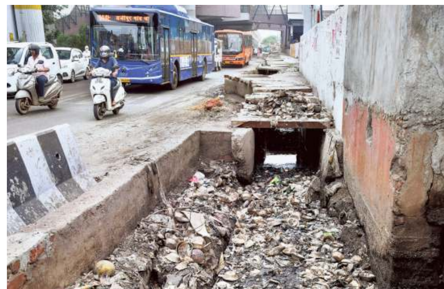
Single-use plastic bags and other trash blocking a drain on GT Karnal Road in New Delhi on Monday. • SUSHIL KUMAR VERMA
